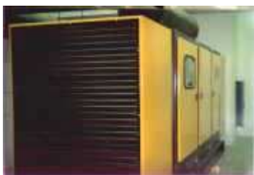
GE 800 Kva City Bank Moscou
